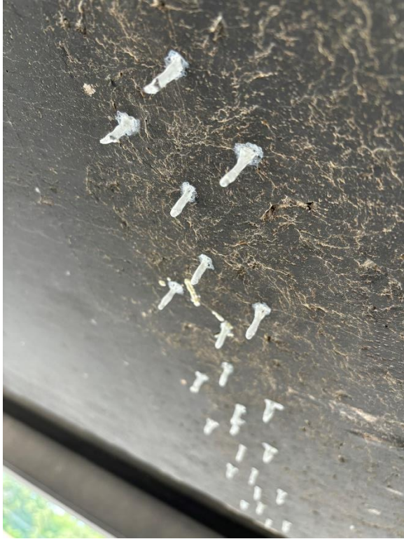
Photo 10: Epoxy that oozed out of the bottom of the bottom flange and re-hardened
