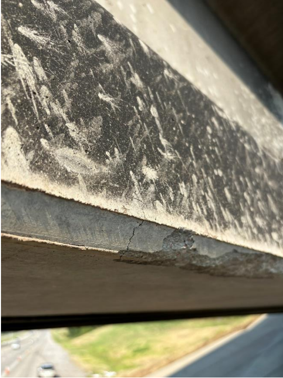
Photo 6: Crack and spall of the bottom flange due to the extreme heat
