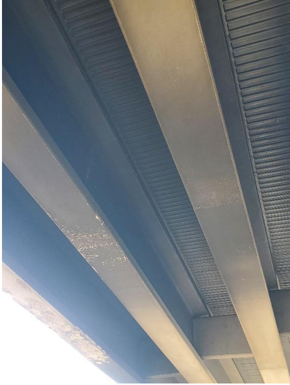
Photo 2: Type J prestressed concrete beams with metal stay-in-place deck forms. These are the three beams that are damaged.
