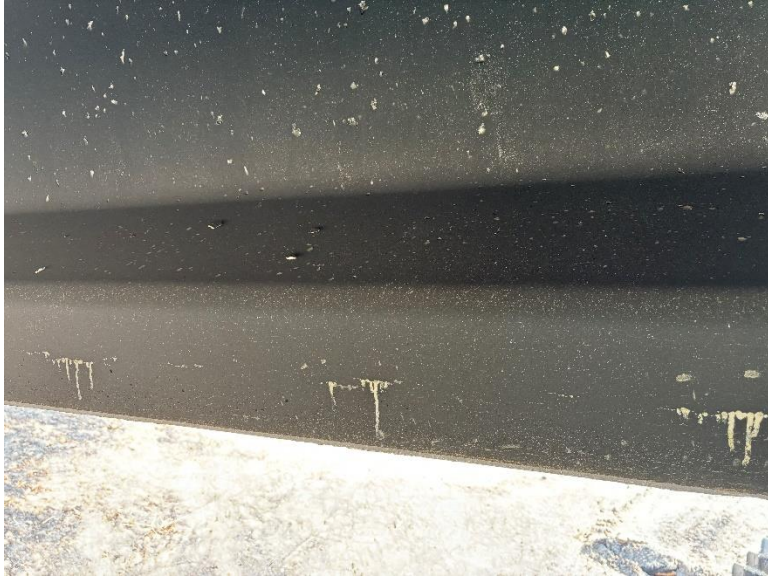
Photo 8: Epoxy coating from the shear stirrups that oozed out of a crack in the interior side of the bottom flange of the exterior beam
