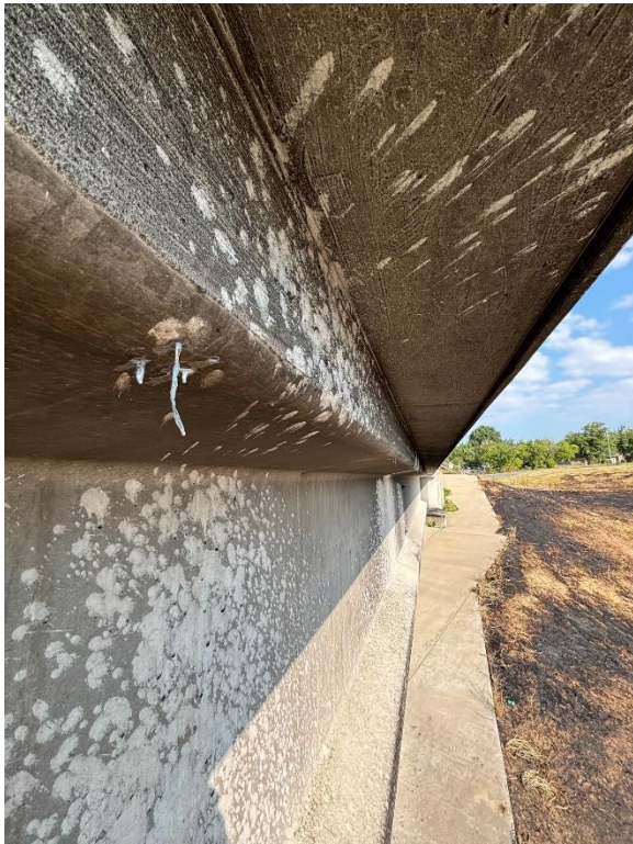
Photo 9: Epoxy that oozed out of the top flange of the exterior beam and re-hardened
