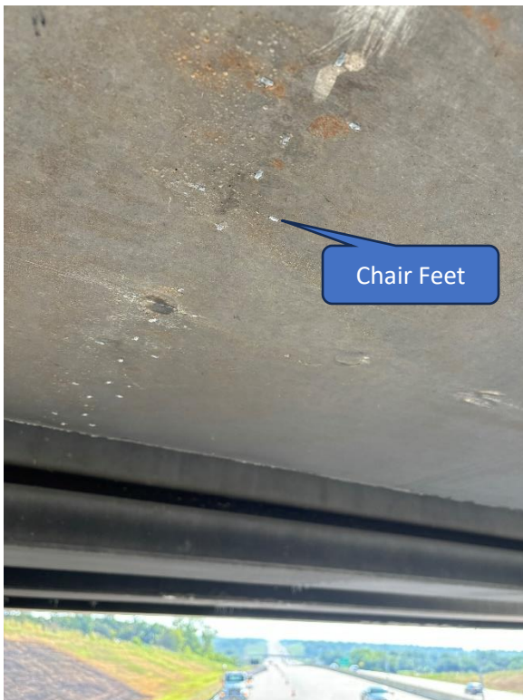
Photo 11: Bottom flange of the fourth beam showing the typical condition of the chairs used in fabrication of the beams
