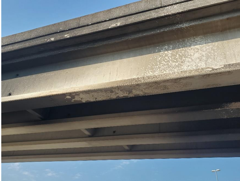
Photo 4: Spalling of both flanges of the exterior beam, exterior face of the deck, and parapet
