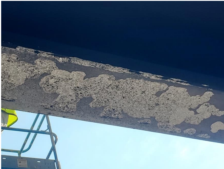
Photo 3: Severe spalling of the concrete in the bottom flange of the exterior beam
