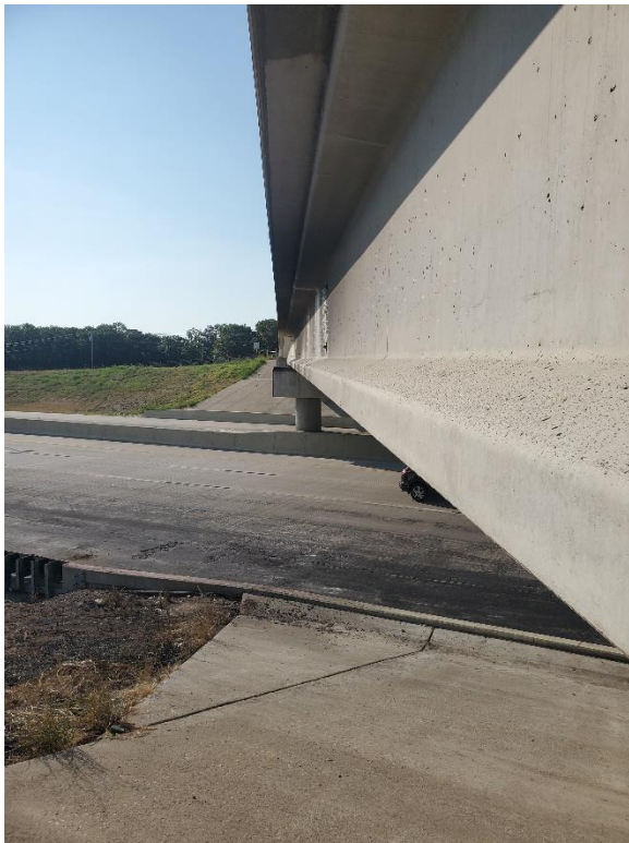
Photo 13: View looking down the length of the damaged exterior beam
