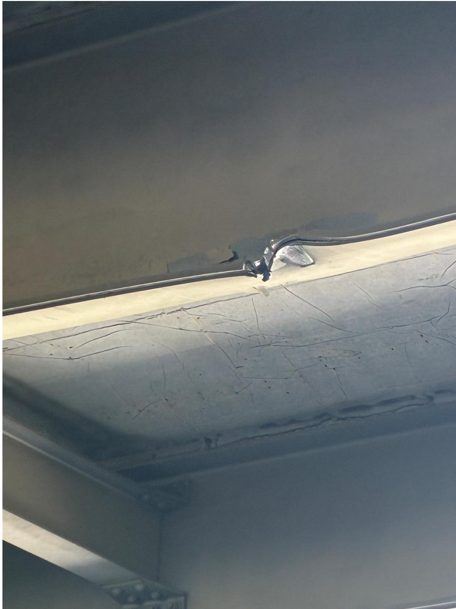
Photo 7: Beam line 11. Torn flange and cover plate
