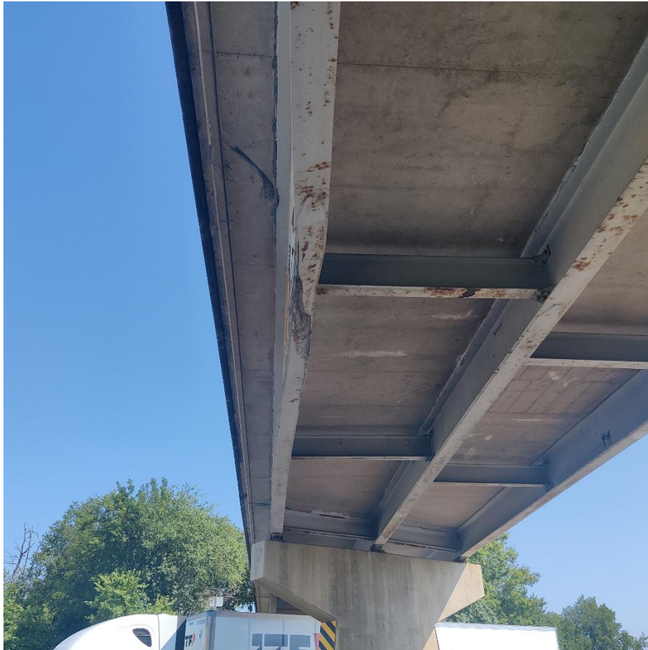
Photo 2: Underside of Bridge. Bent flange and scrape marks from impact
