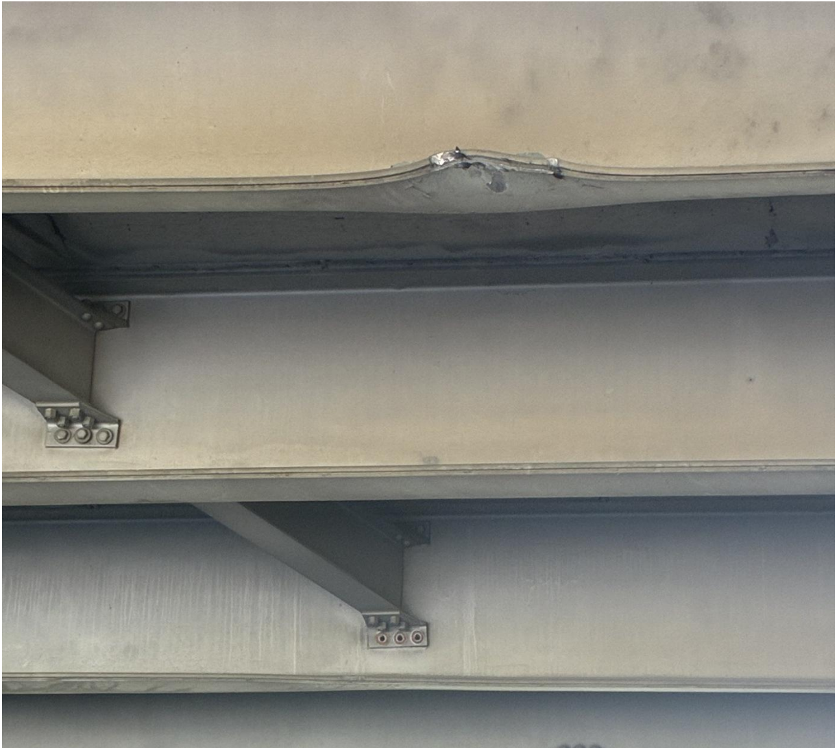
Photo 4: Beam line 5. Bent flange and cover plate
