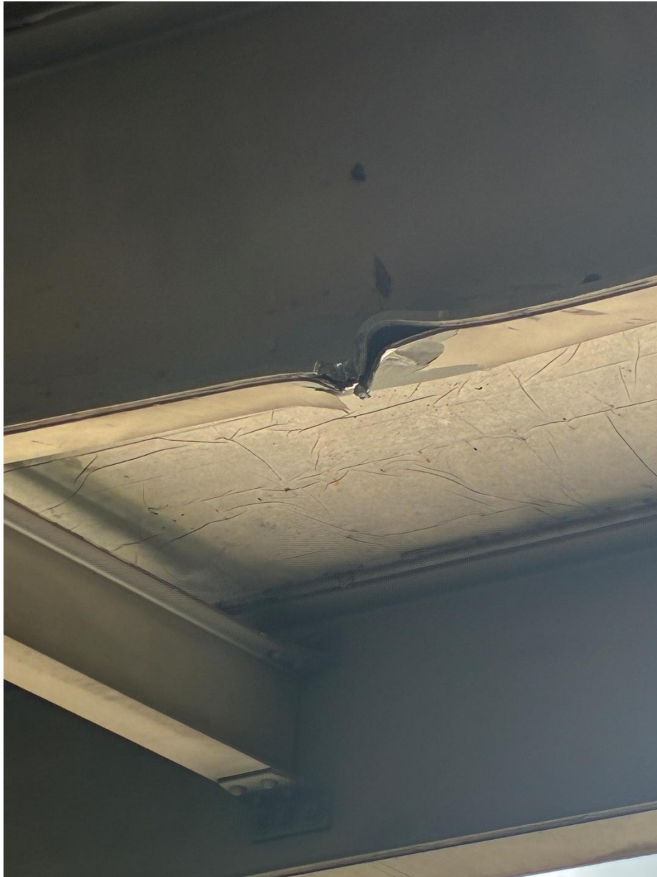
Photo 8: Beam line 13. Torn flange and cover plate
