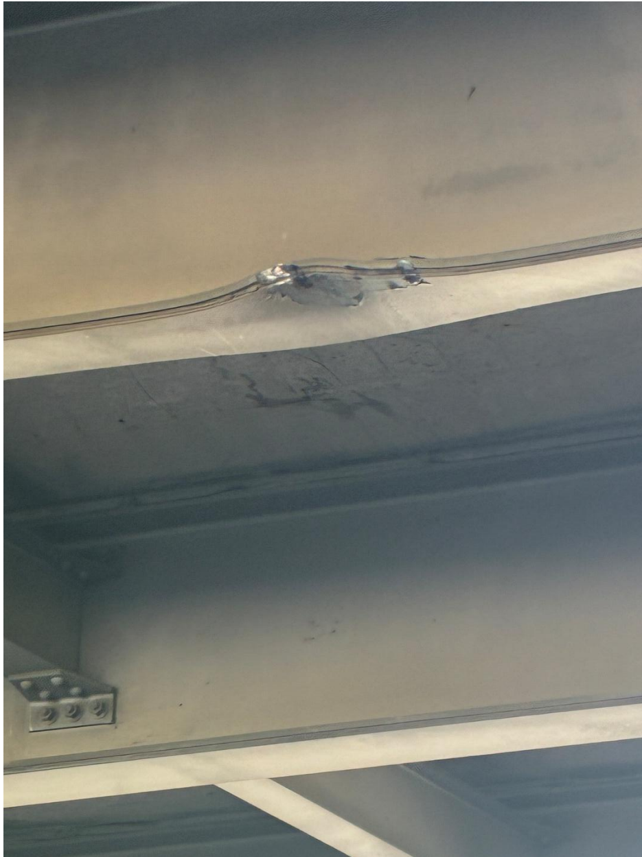
Photo 6: Beam line 9. Bent flange and cover plate
