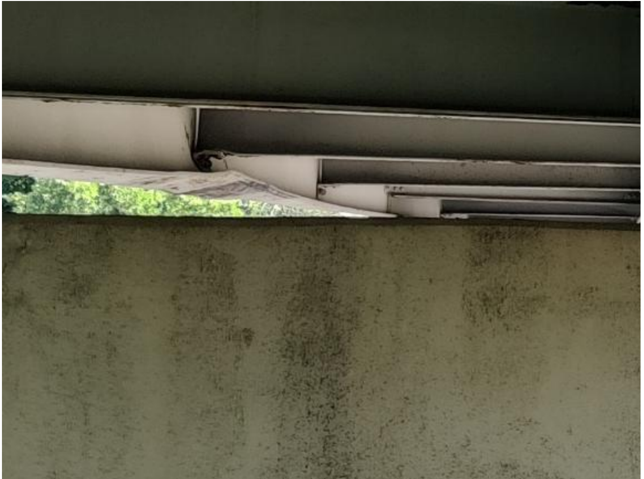
Photo 3: Beam flange and web bent due to impact
