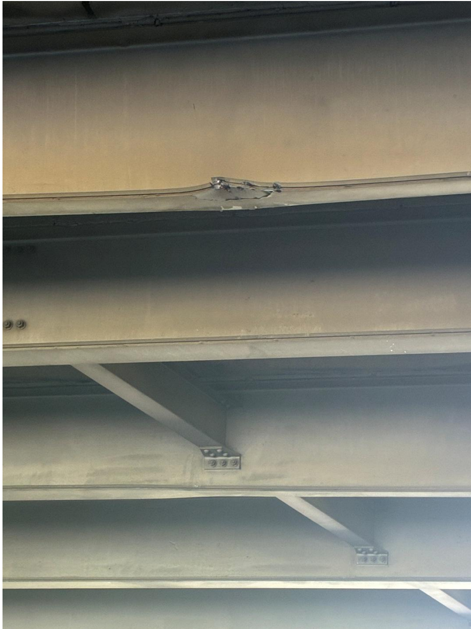
Photo 5: Beam line 7. Bent flange and cover plate with a minor tear
