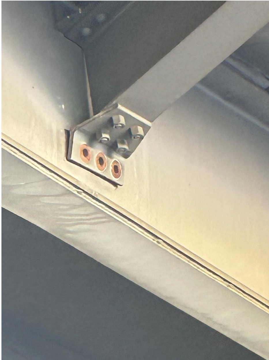
Photo 9: Diaphragm bolts missing between beams 5 and 6
