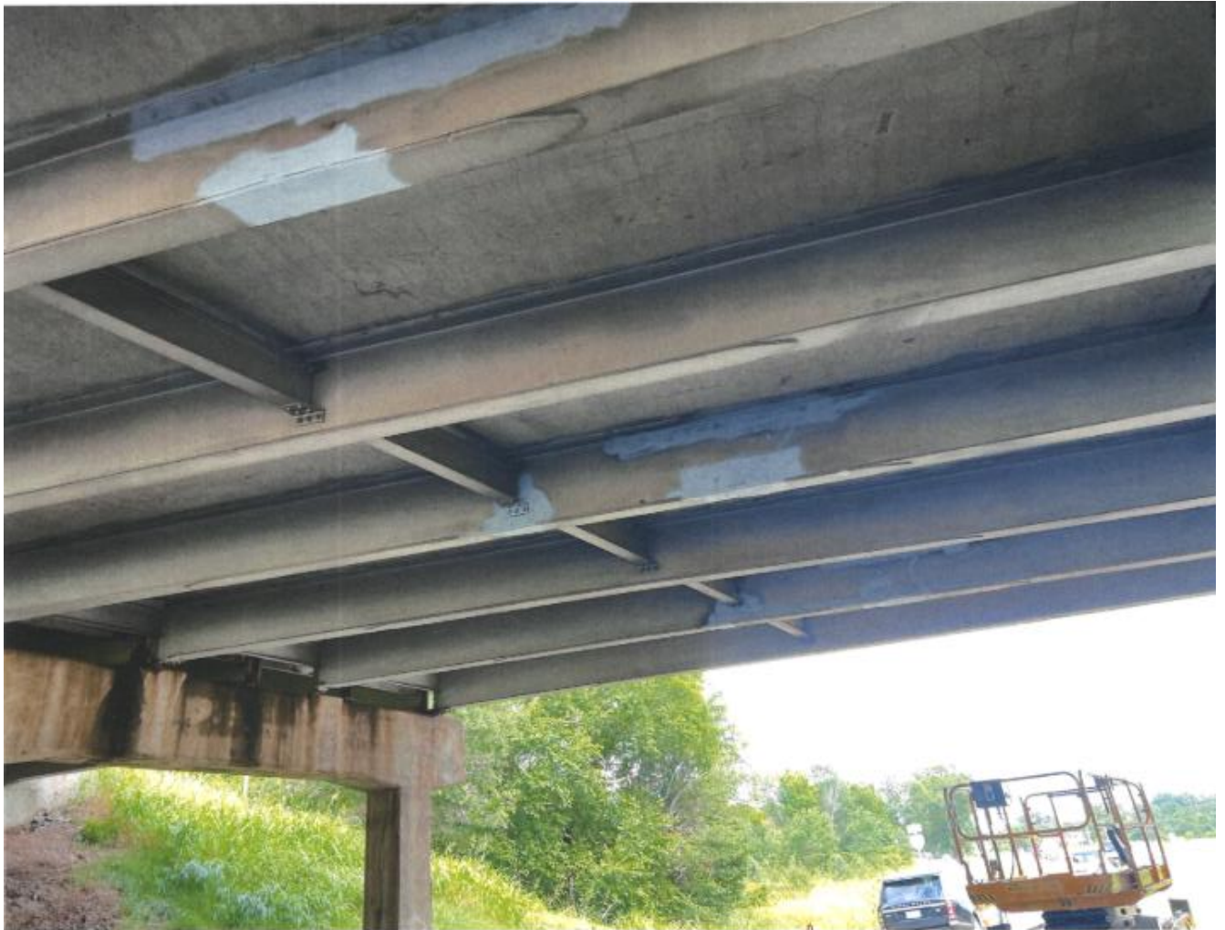
Photo 10: Underside of deck showing areas of repair
