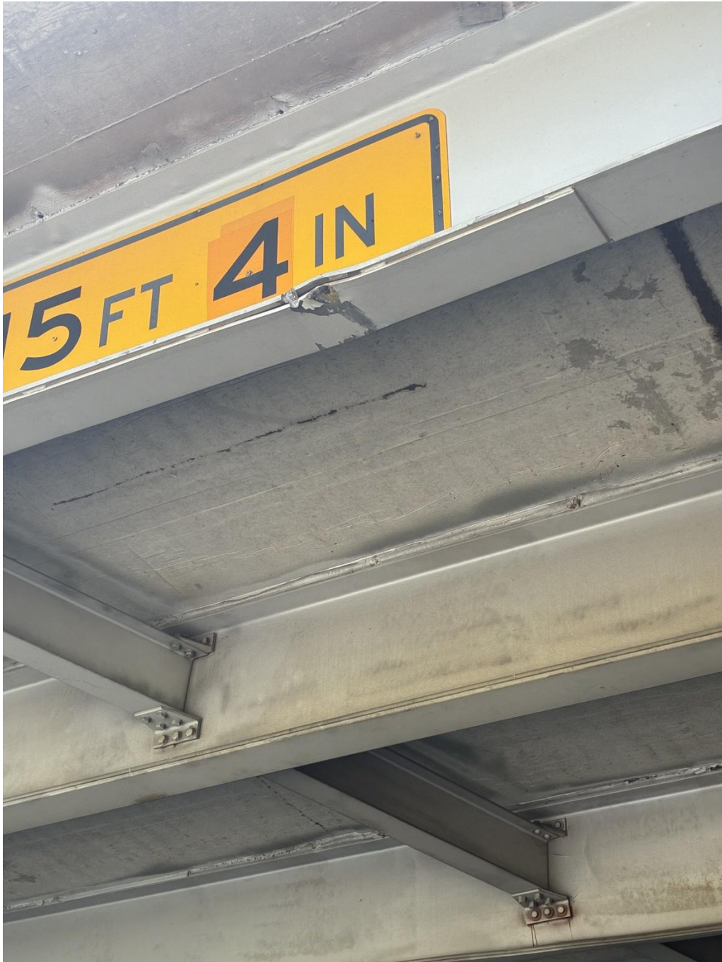
Photo 2: Beam line 1. Bent flange and scrape marks from impact
