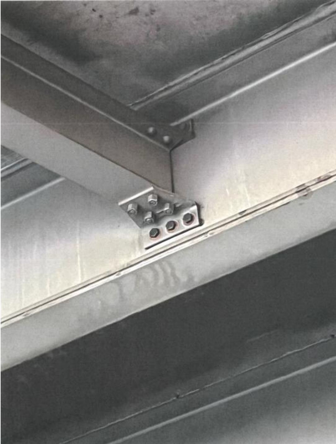
Photo 12: New diaphragm bolts
