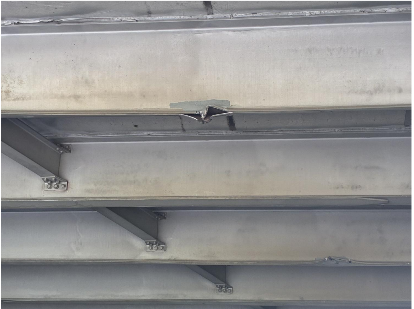
Photo 3: Beam line 3. Torn flange, cover plate and bent web
