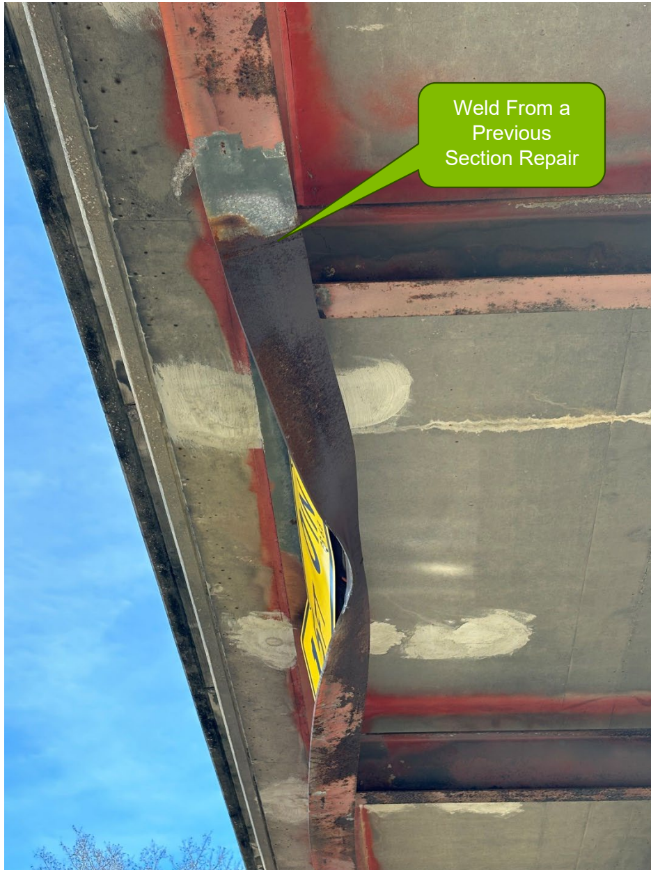
Photo 7 –Previous Section Repair with Full Penetration Weld
