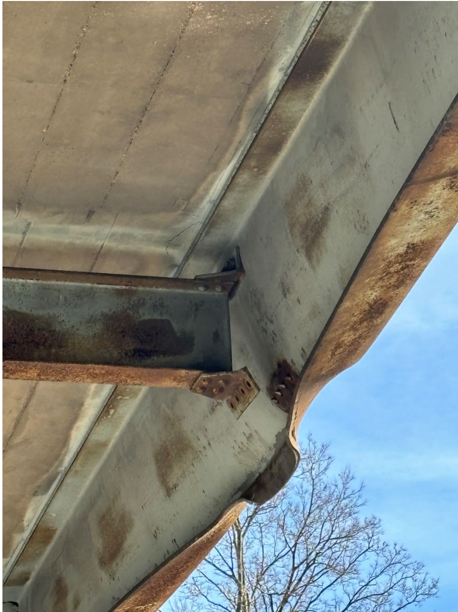
Photo 6 - Damage to the Diaphragm Connections
