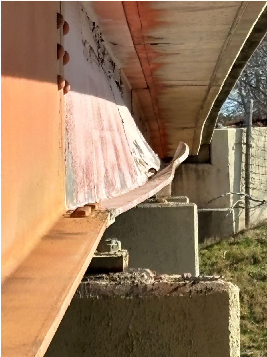
Photo 3 - West Exterior Beam Damage
