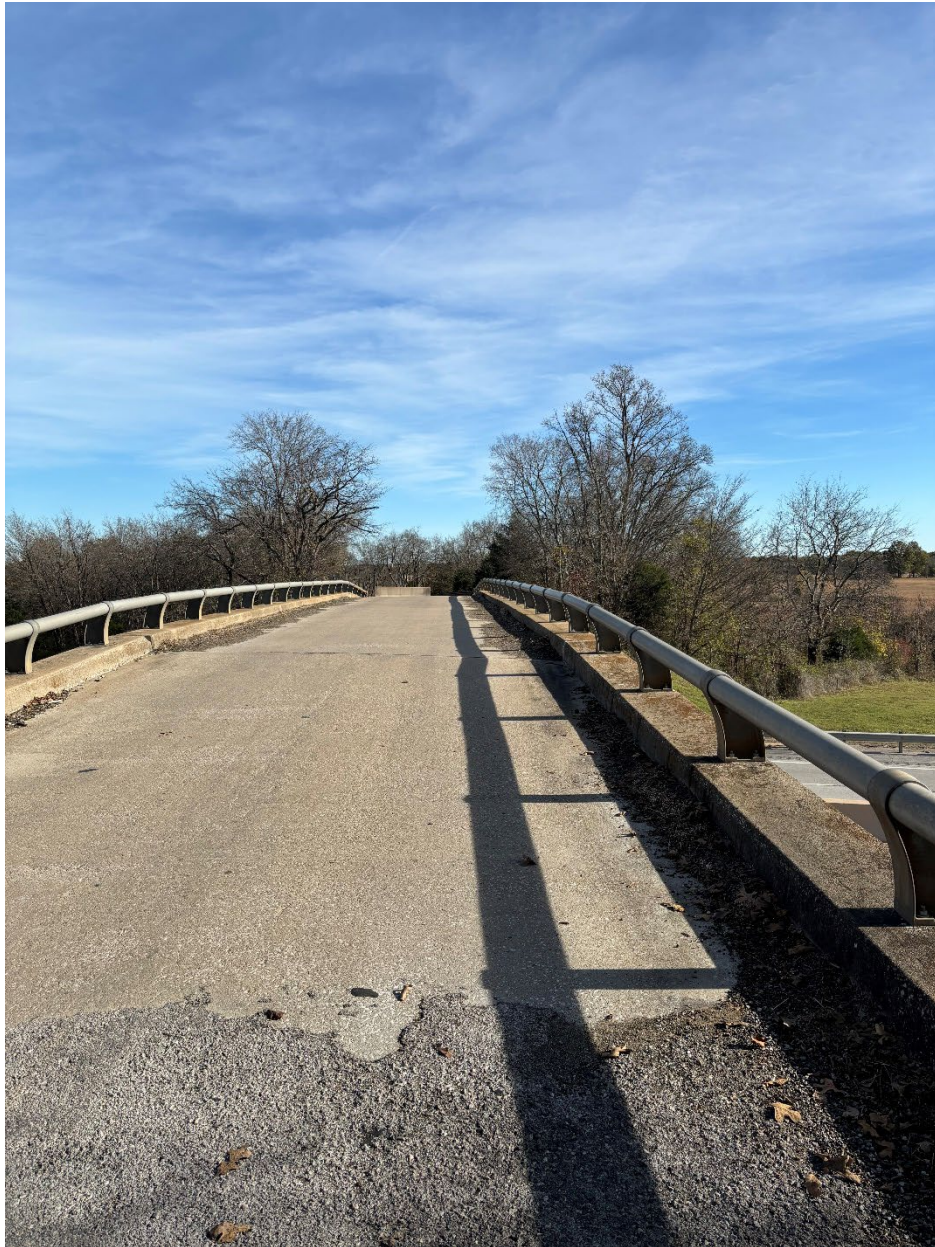
Photo 7 – Deck Following Impact
