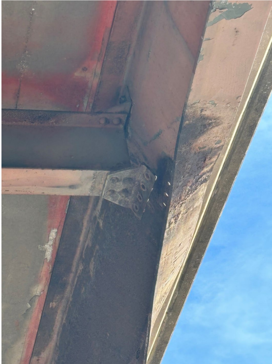
Photo 5 - Damage to the Diaphragm Connections
