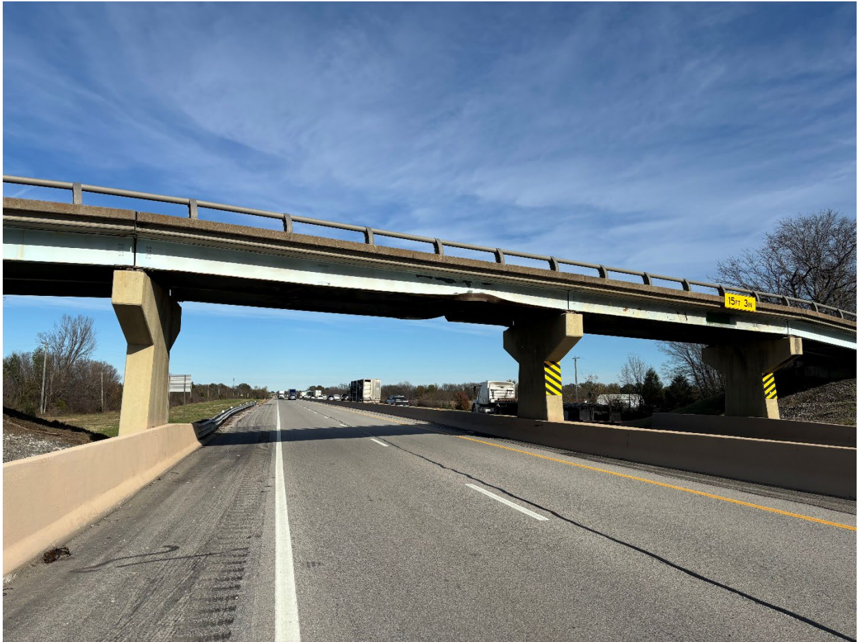
Photo 2 - Damage from Vehicular Impact Over the Inside Lane
