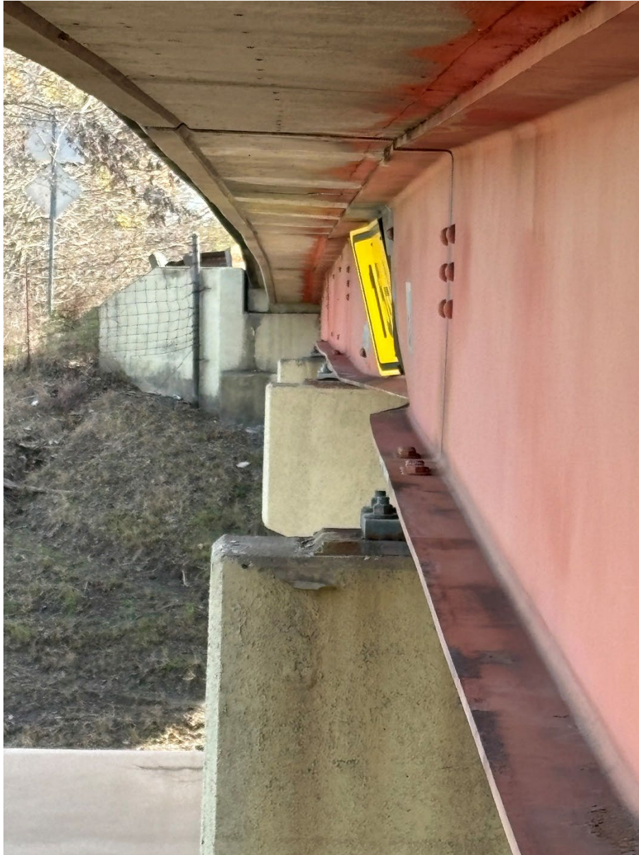
Photo 4 – East Exterior Beam Damage
