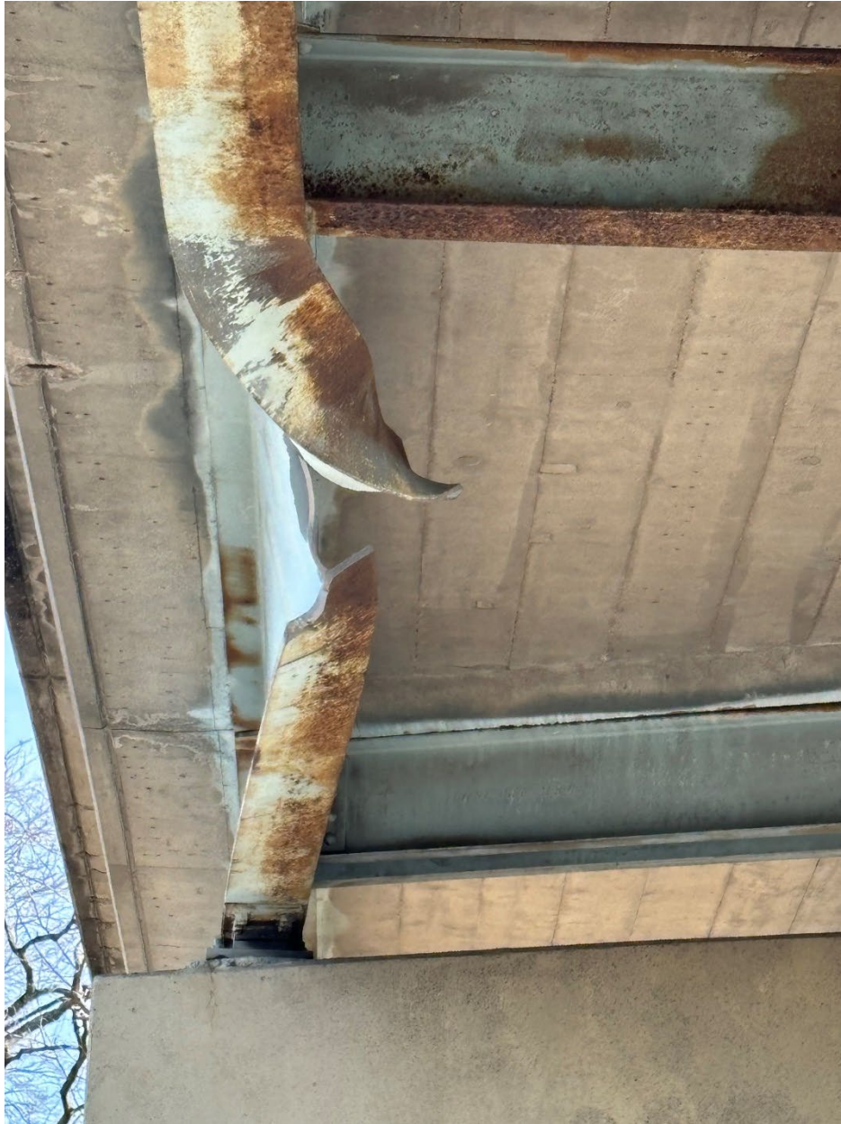
Photo 5 - Tearing of the East Exterior Beam
