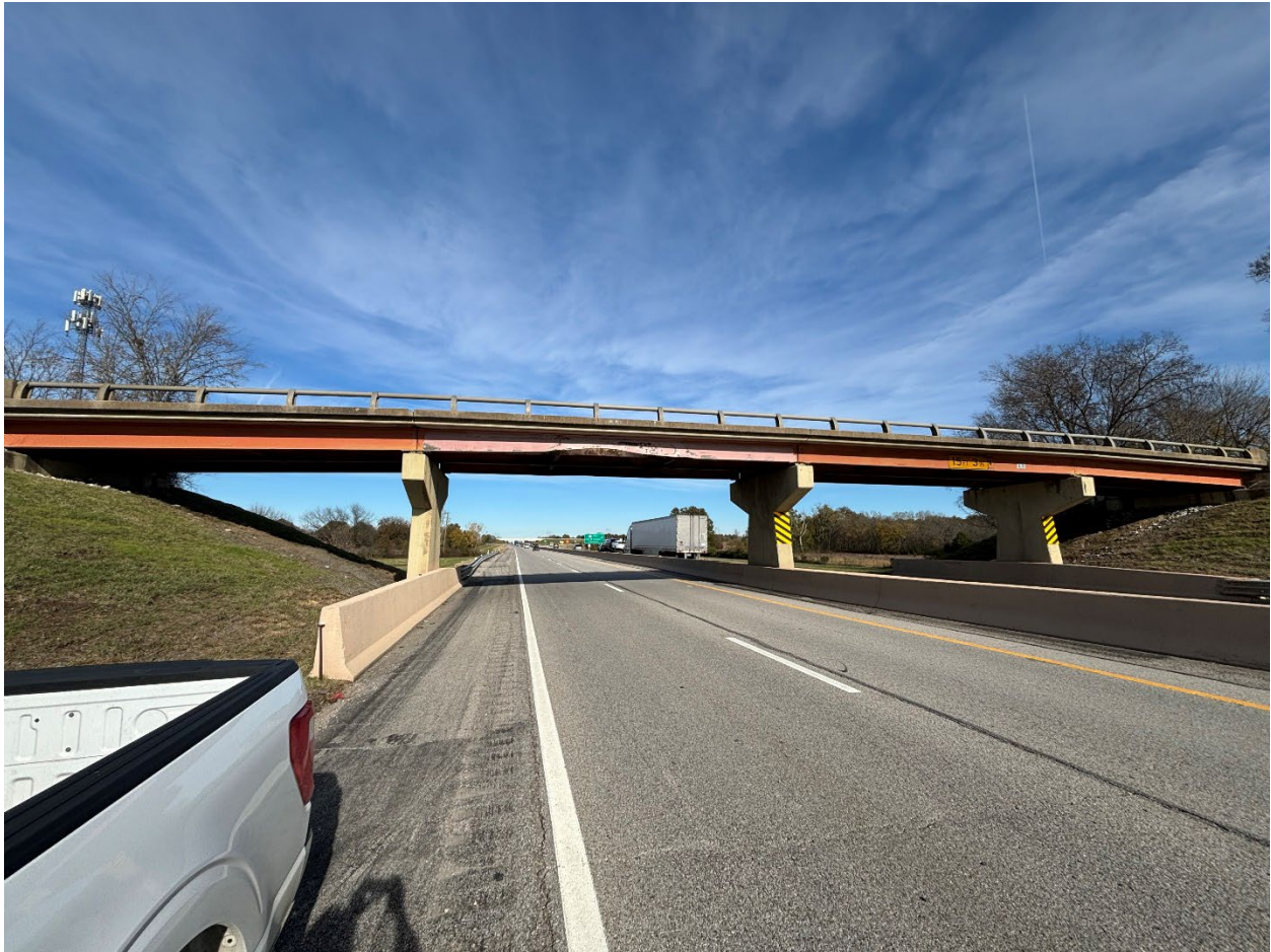
Photo 2 – Location of the Damage from Vehicular Impact Near Center of Span
