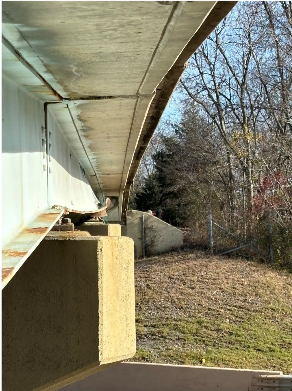
Photo 3 - West Exterior Beam Damage
