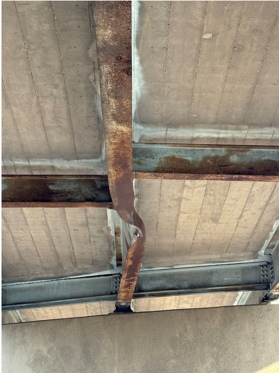
Photo 4 - Interior Beam Damage
